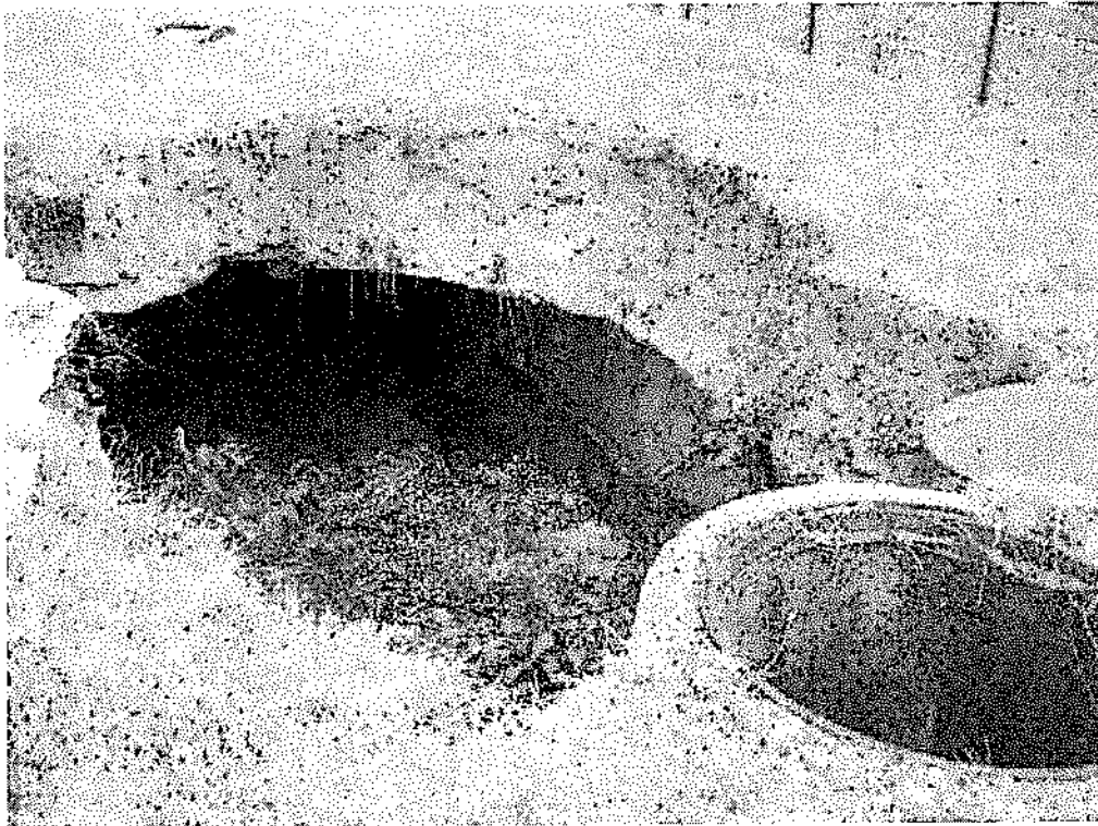
VIEW OF COLLAPSED UNDERGROUND FILTRATION CELL
