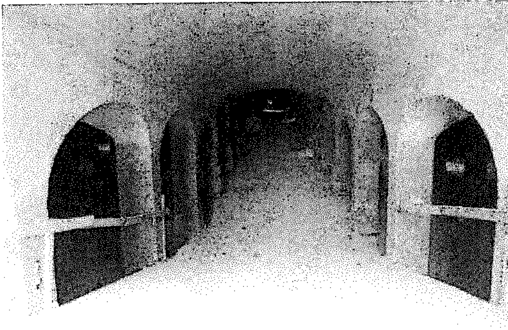
INTERIOR VIEW OF UNDERGROUND FILTRATION CELL
